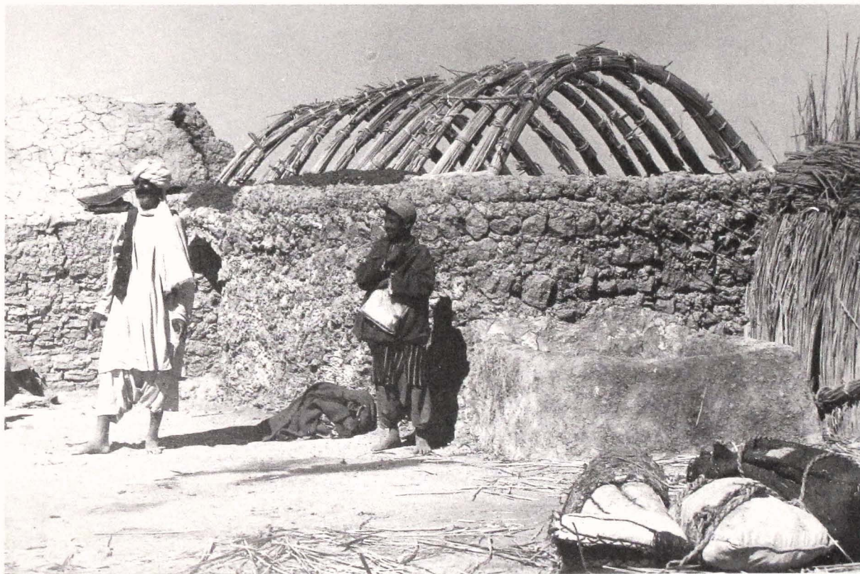
34. A building of bundled reed vaulting embedded in pakhsa walls under construction in Seistan, north of Zaranj.
